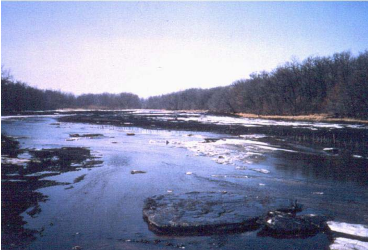
Image 1. Root River at Stewartville, MN after excavation of an over-wide and over-deep channel.
